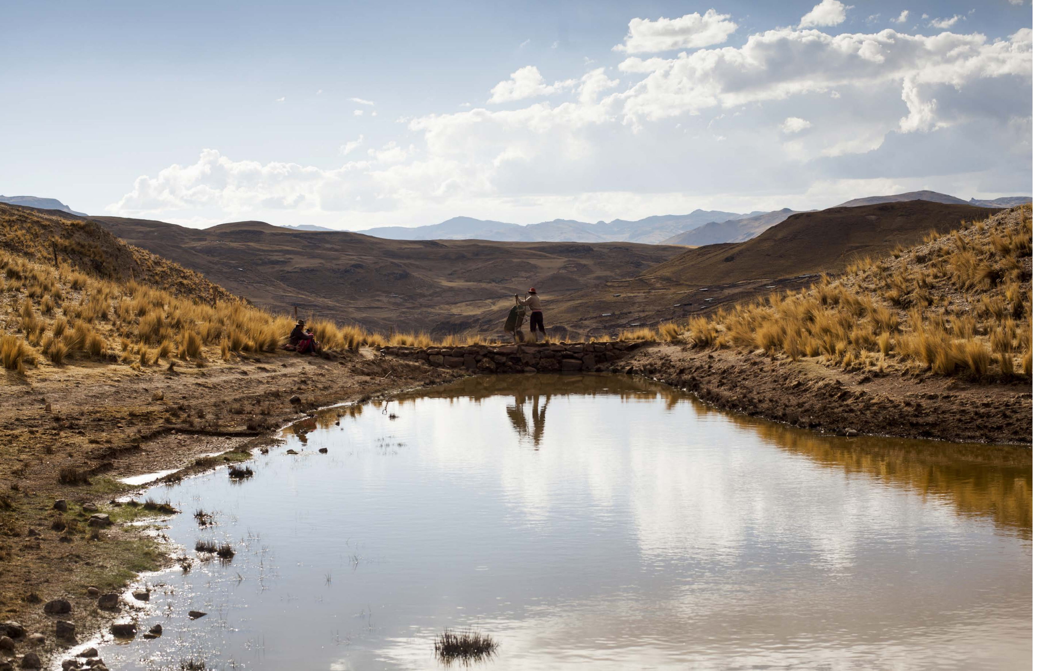
➔ Necessary maintenance. Community members Brigida Consonne and Clemente Choquipuma work on the reinforcement of the dam of a qocha in Quilinuara. The positive effects of this lake are evident in land below, where small springs have been recovered.
